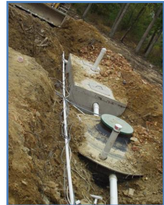
Alternative On-site Sewage Disposal System
