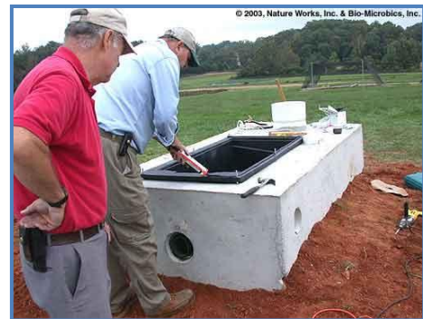
On-site Sewage Disposal System
