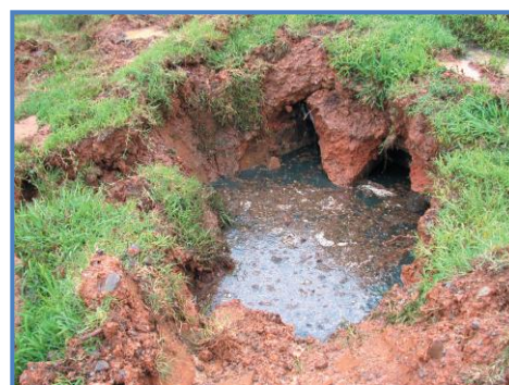
Failed Septic System
